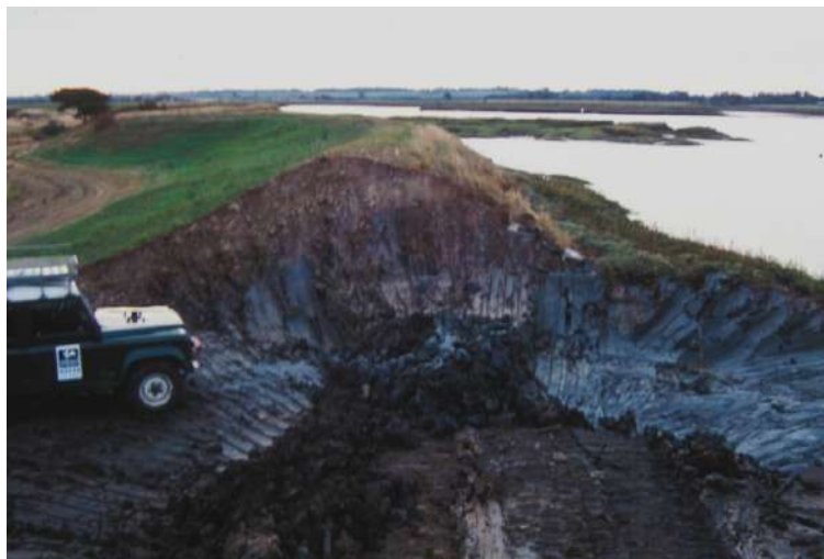
FIGURE 35: ABBOTTS HALL BREACH (2002)
